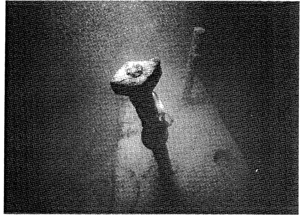
WB-89-256 L 183 NW cxg Bolt in span
